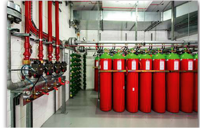
Fire Suppression System
