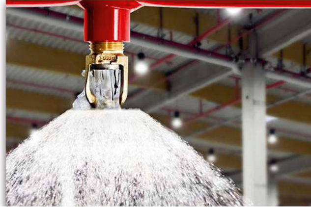
Fire Sprinkler System
