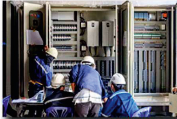
Electrical Panel Services
