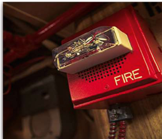
Fire Alarm System
