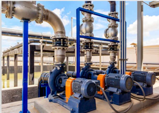
Pipe lines And Pumps
