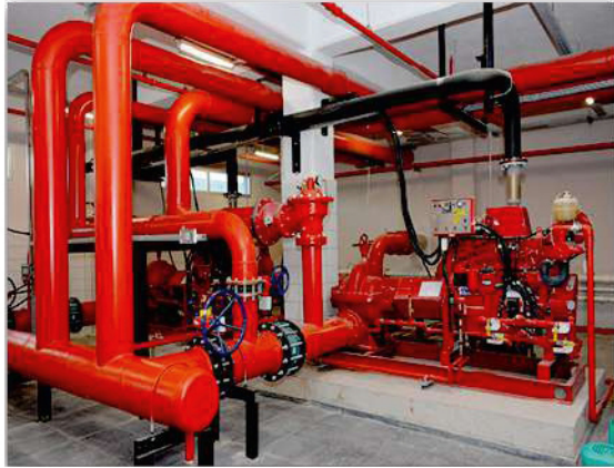
Fire Hydrant System
